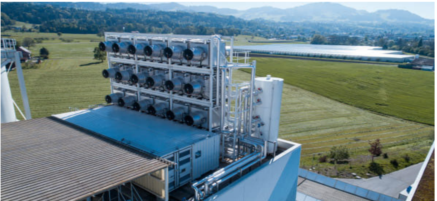
Climework's facility in Zurich. [Photo: Julia Dunlop/courtesy Climeworks]
